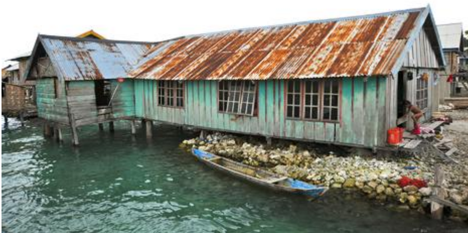
A corrugated iron roof rusting in a marine environment
