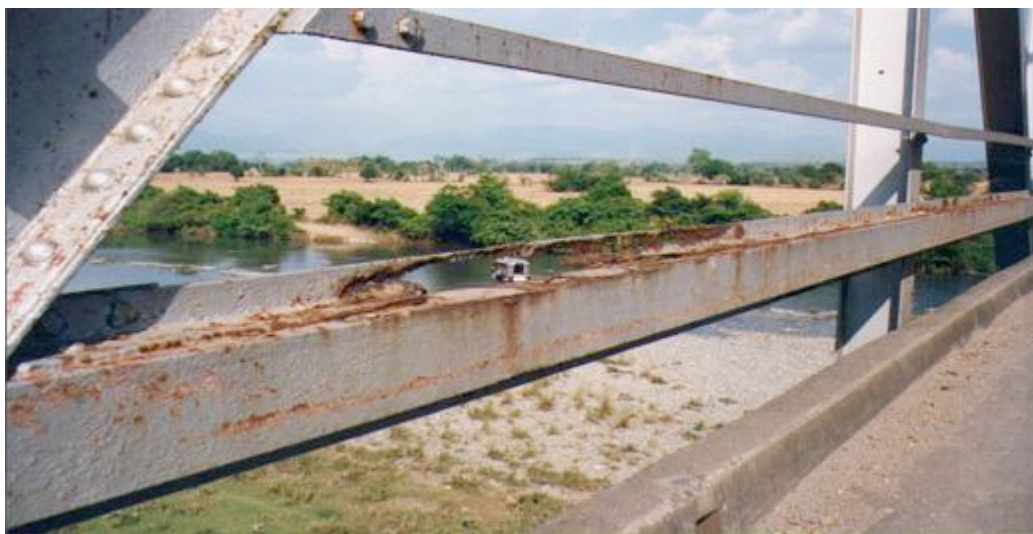
A severely corroded bridge suggests great danger!
